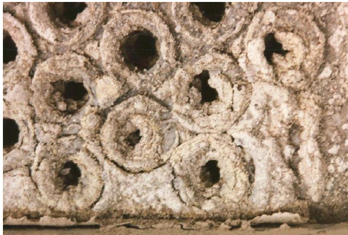
FIGURE 6. AMMONIA SALTS ON CONDENSER TUBE SHEET
