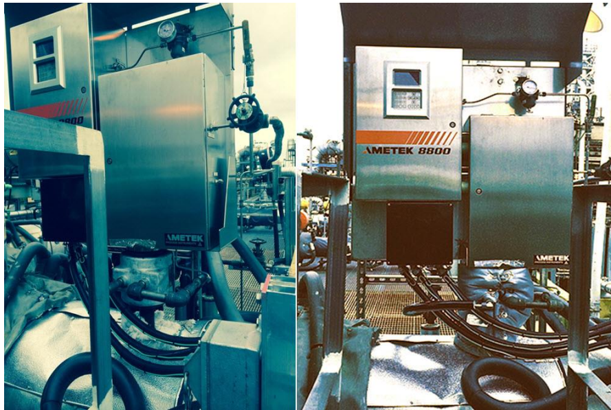
FIGURE 8. FIELD TRIAL PBF PAULSBORO REFINERY
